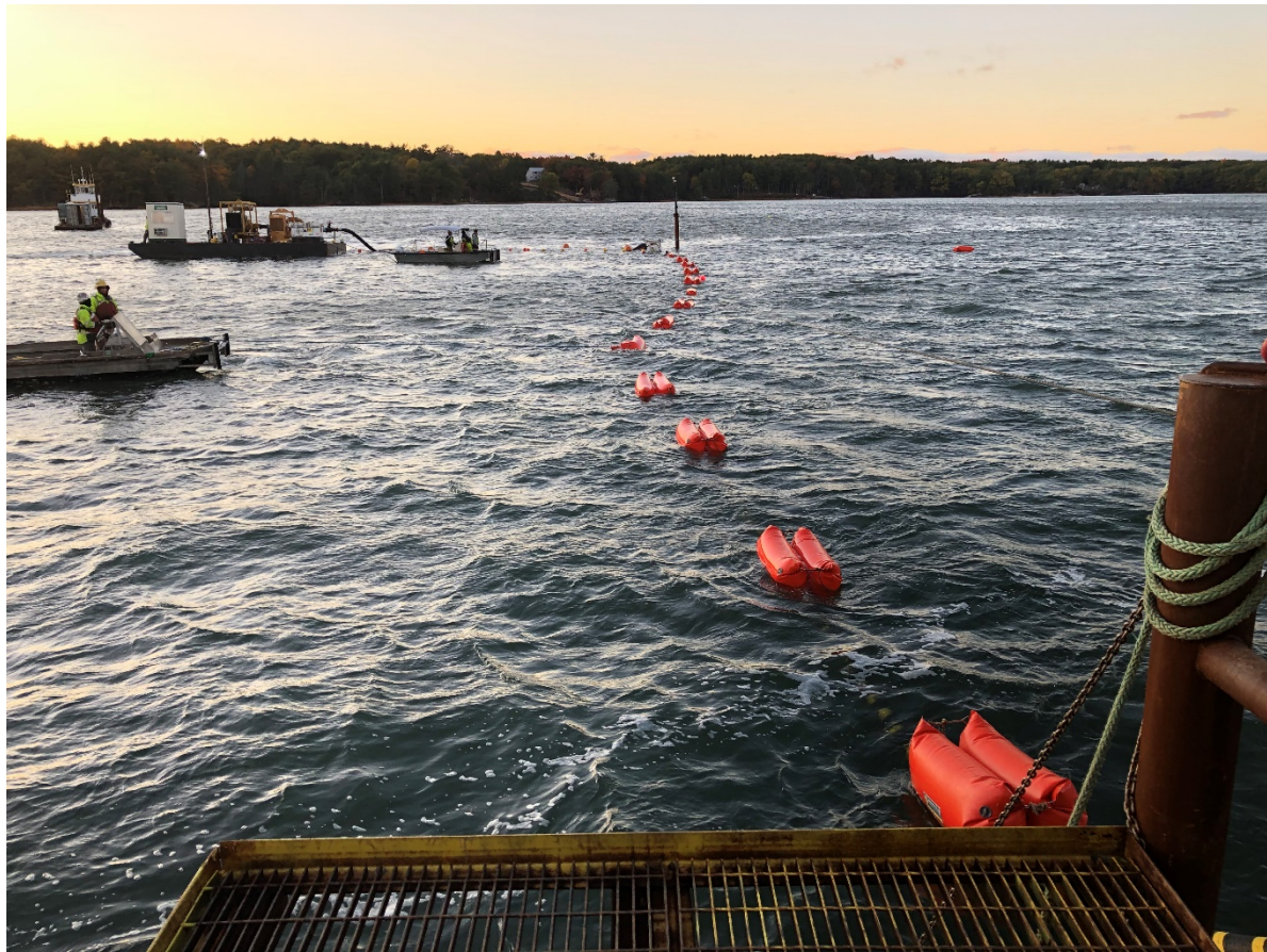
Cable and float bag setup from work platform back of barge. Diver barge and tug (upper left), pump barge and work boat (upper center), work boat (left).
